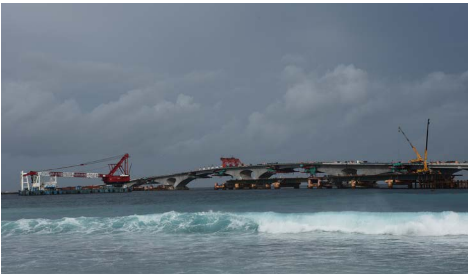
Figure 2. Construction work on the China-Maldives Friendship Bridge. Photograph by R. Michael Feener.
