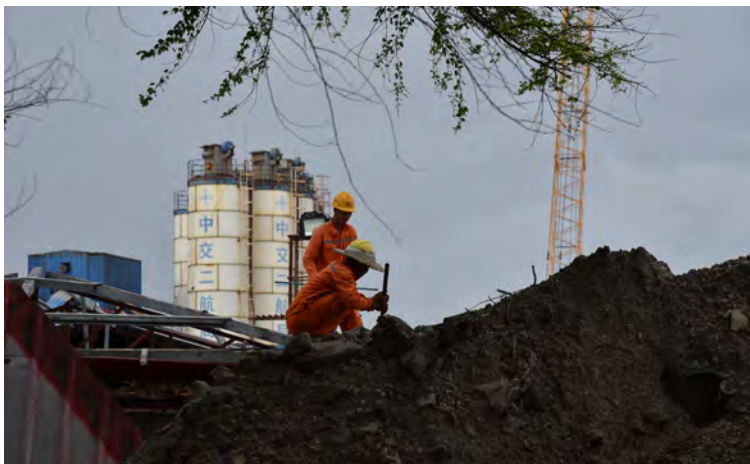
Figure 8. Foreign labor at work on the construction of the Sinamale' Bridge. Photograph by R. Michael Feener.
